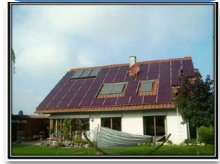
Residential Rooftop PV system
