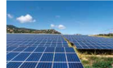
PV Power Plant
