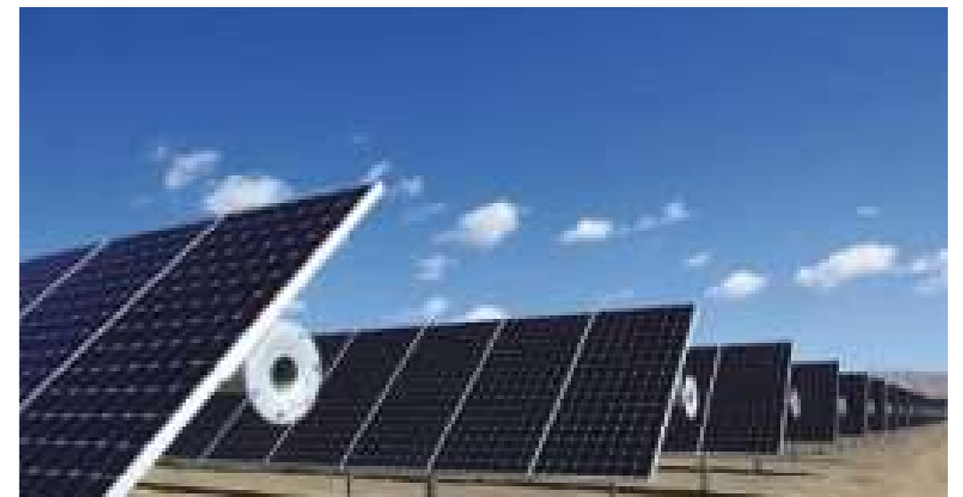
4.3 MW PV Power Station in Puglia Italy
