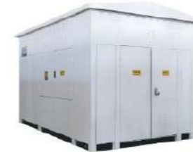
Photovoltaic split transformer
