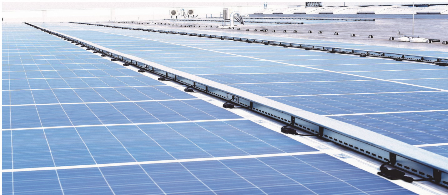
Rooftop installation DAS Energy Headquarters
