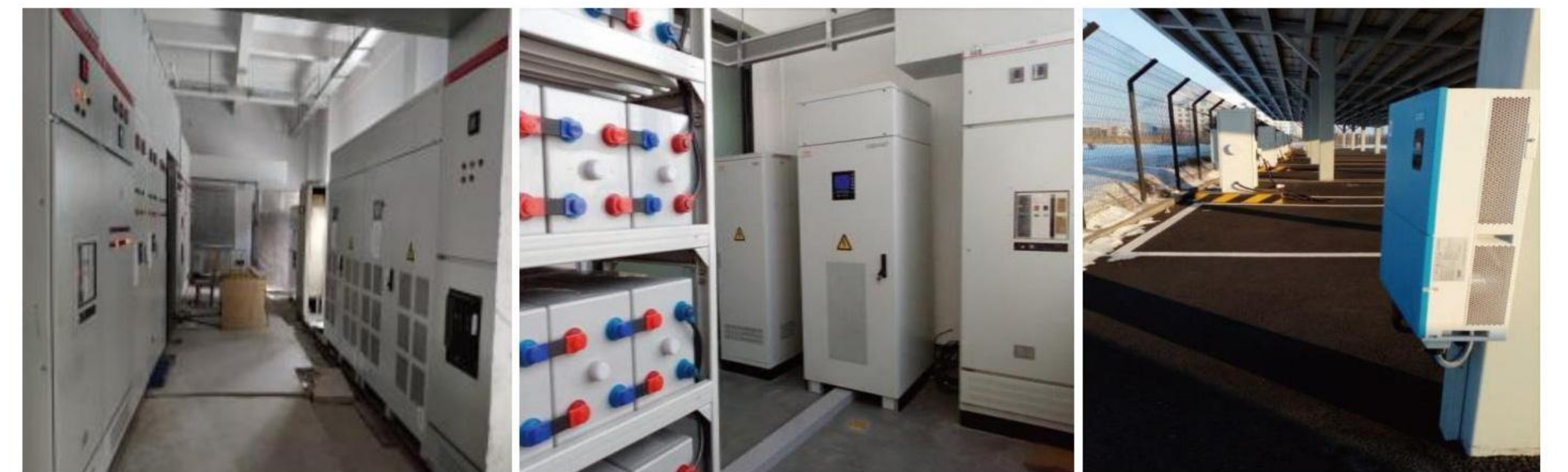
▶ BESS for EV Charger Station in Harbin
