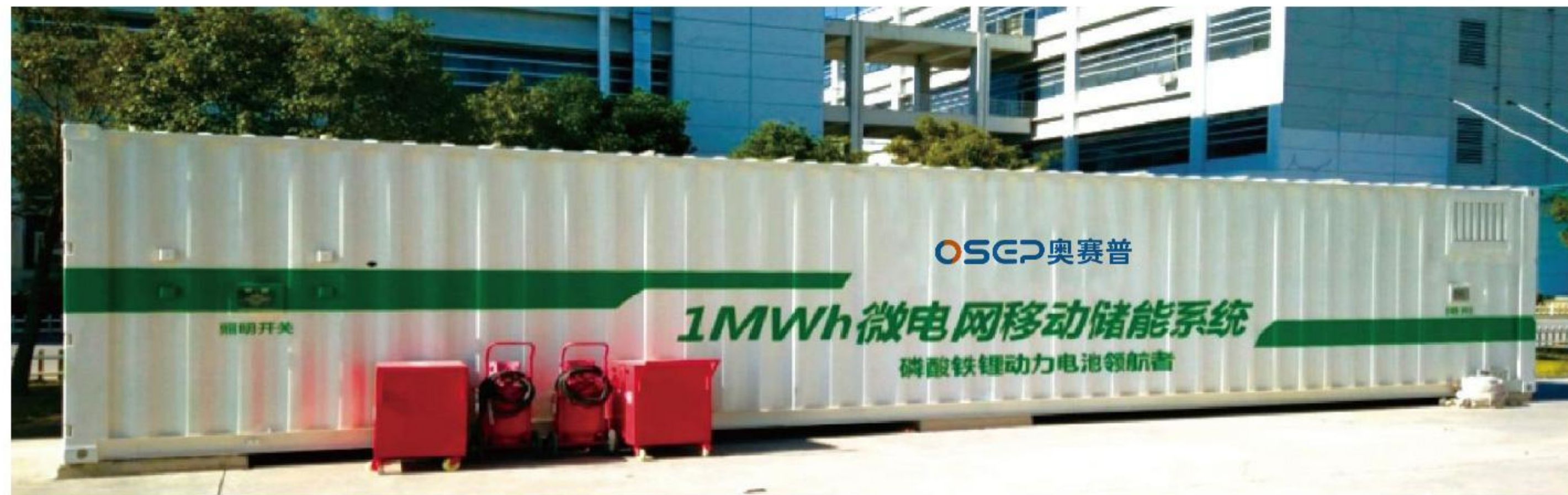
▶ 3MW/12MWh BESS Demonstration Project in Shenzhen
