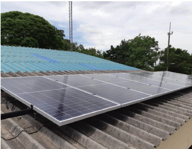
Thailand, 3kW corrugated roof mounting
