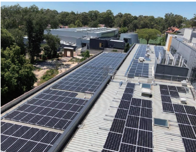
Australia, 200kW metal roof mounting
