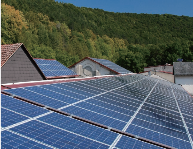
Germany, 60kW metal tile roof mounting
