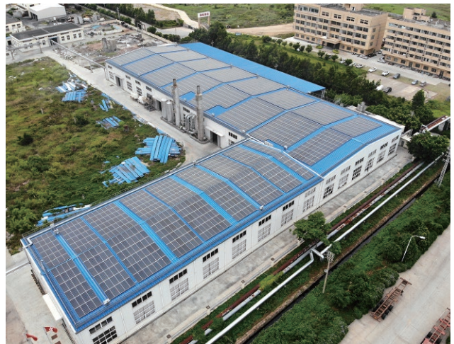
China, 800kW factory metal roof mounting
