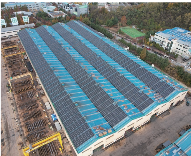
South Korea, 2.5MW factory metal roof mounting
