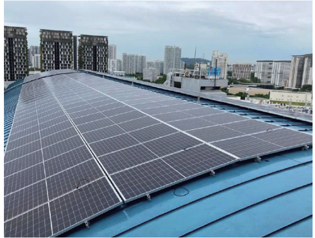
China, 120kW curve metal roof mounting
