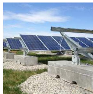
2 MW - Maynard Landfill Massachusetts
