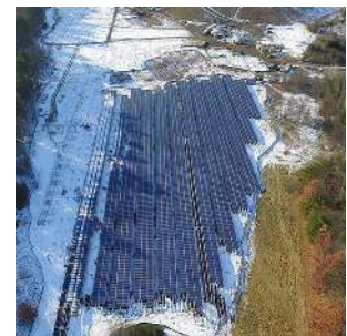
3.2 MW - Hudson Landfill Massachusetts
