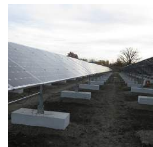
1.2 MW - Marysville Michigan
