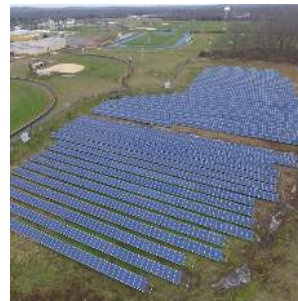
2 MW - Plumsted School New Jersey
