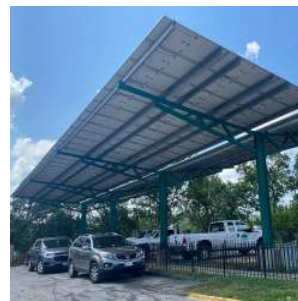
1 MW - WASHINGTON DISTRICT OF COLUMBIA
