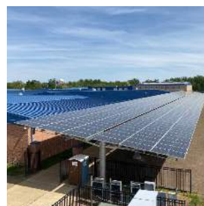
560 kW - SOMERDALE NEW JERSEY
