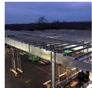
1.2 MW - EAST WINDSOR CONNECTICUT
