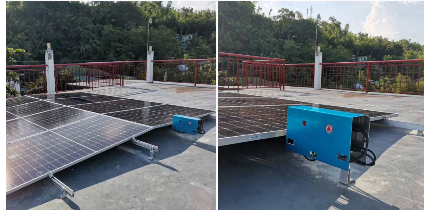
CASE STUDY: 6kW Grid-tied System in the Philippines
