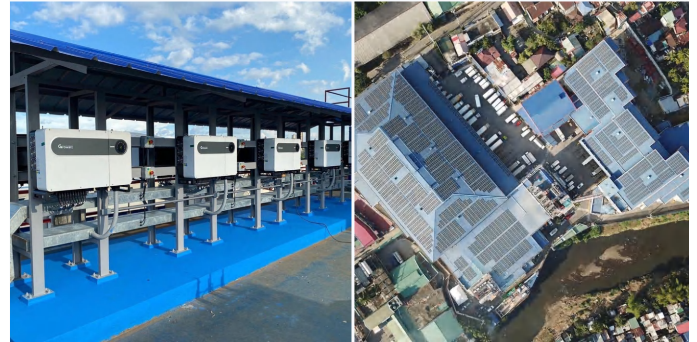
CASE STUDY: Philippines with 1.2MW solar installation.
