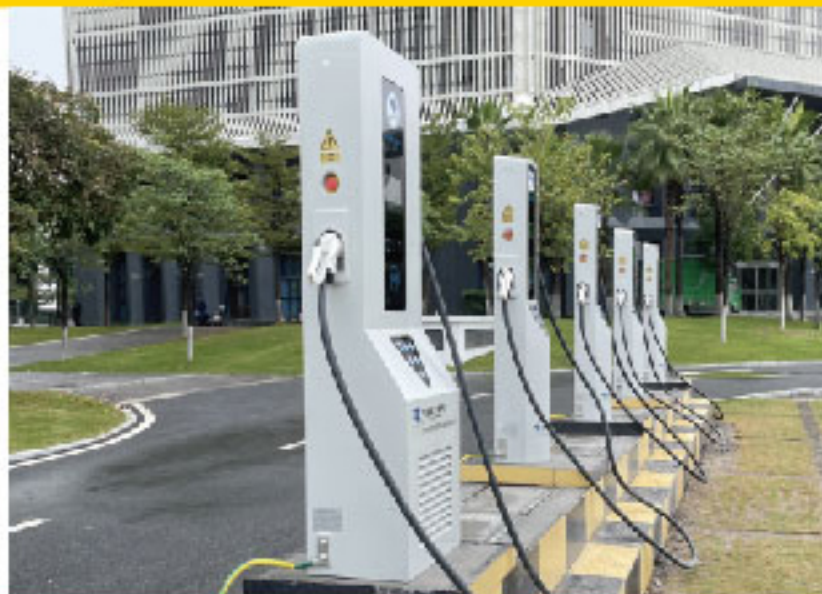
电动汽车超级充电站 EV Supercharging Station
