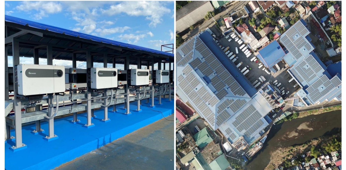
CASE STUDY: Philippines with 1.2MW solar installation.
