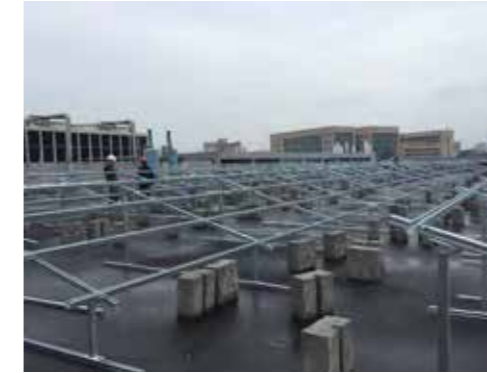
Project Location: Tuas, Singapore Capacity: 1MWp Completion Year: 2017 Type: RC Roof Mounted
