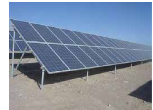
Project Location: USA Capacity: 2.5MWp Completion Year: 2015 Type: Ground Mounted
