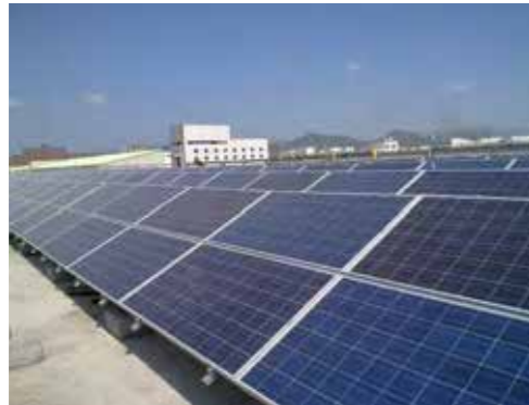
Project Location: Shanghai, China Capacity: 60MWp Completion Year: 2018 Type: Concrete Roof Mounted
