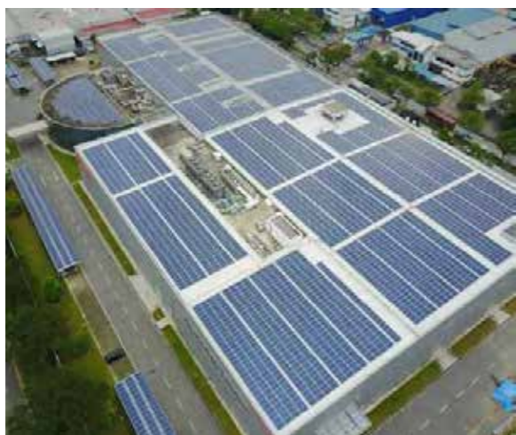
Project Location: Singapore Capacity: 1.6MWp Completion Year: 2017 Type: Metal roof Mounted
