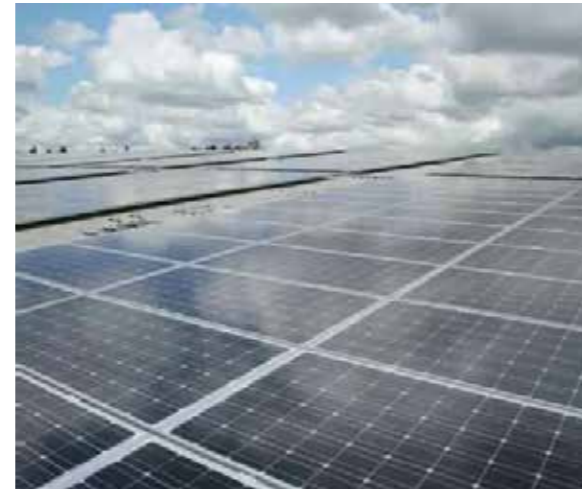
Project Location: Klang, Malaysia Capacity: 426kWp Completion Year: 2016 Type: Metal roof Mounted
