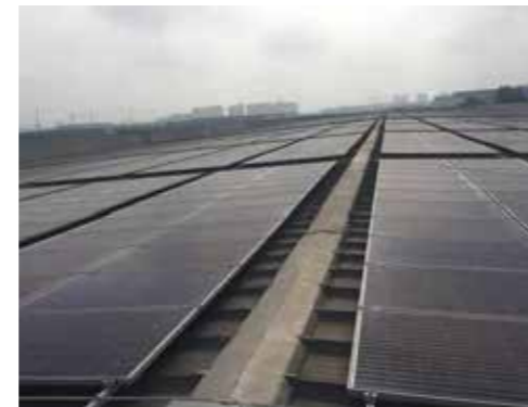
Project Location: Shiga-ken, Japan Capacity: 2MWp Completion Year: 2015 Type: Metal Roof Mounted
