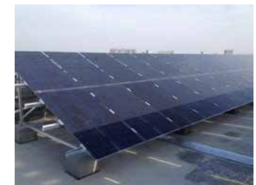
Project Location: Cebu, Philippines Capacity: 2.5MWp Completion Year: 2017 Type: RC Roof Mounted
