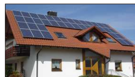
Off-grid home solar system
