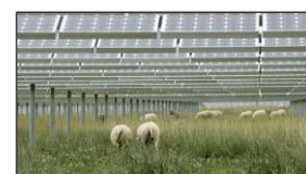
Farm solar generation system
