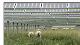
Farm solar generation system
