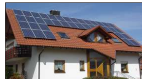
Off-grid home solar system
