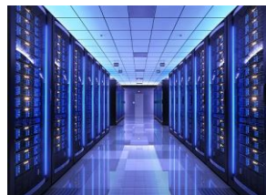
UPS & IDC Datacenter
