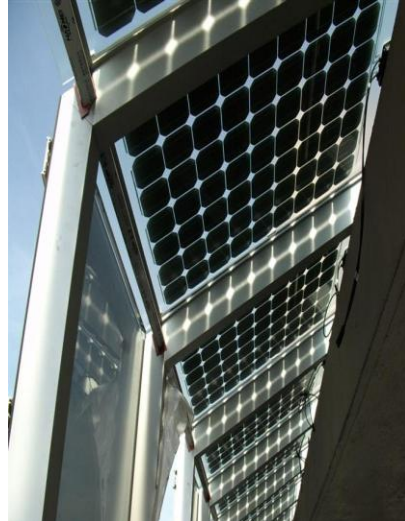
☀️ Shanghai People's Square Solar System
