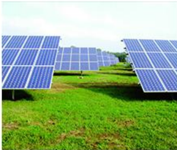
BAVARIA (DE) ESPSA 180W, 1.5MW
