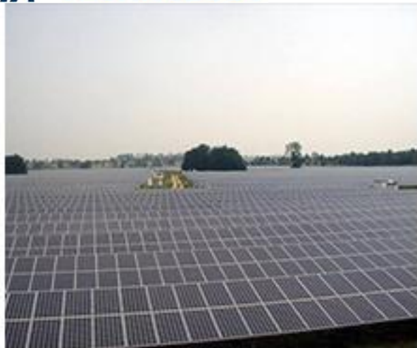
THAILAND ESPSA 190W, 8MW
