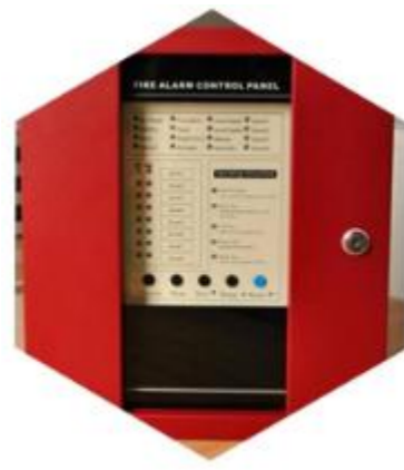
Fire alarm system
