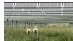
Farm solar generation system
