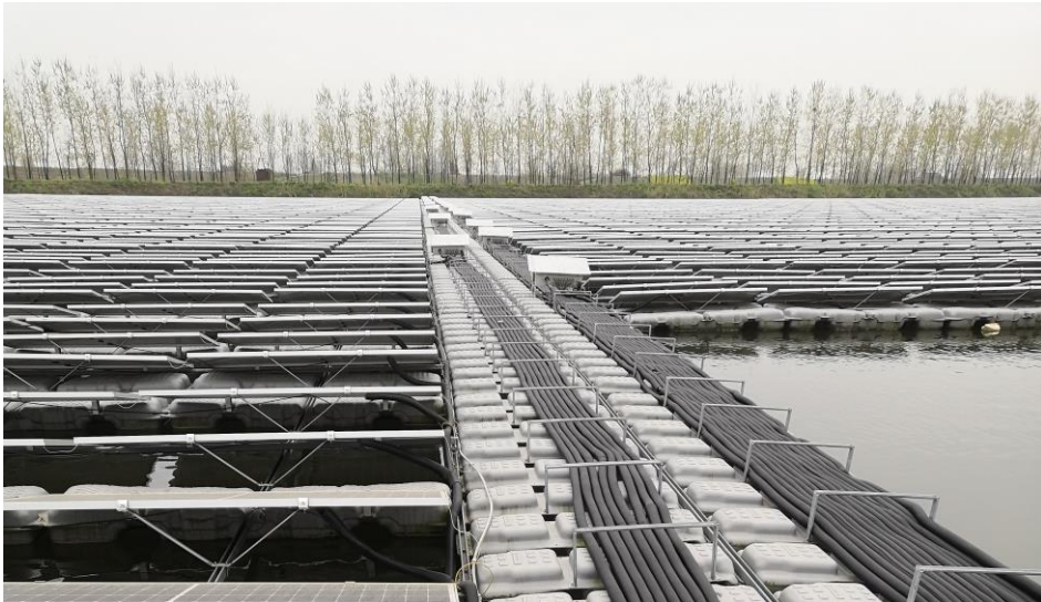
Sidewalk floater for cable inside island
