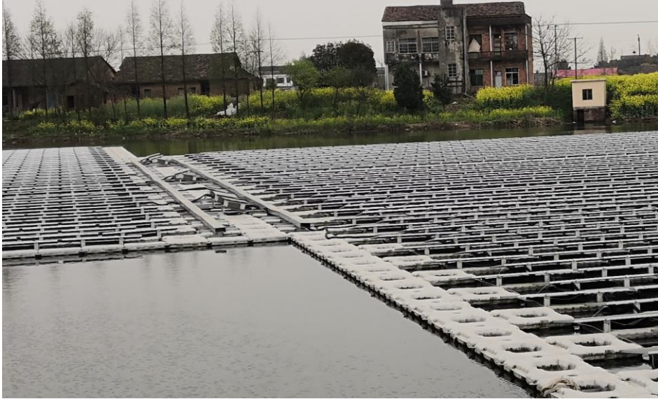
Equipment floater for cable inside island
