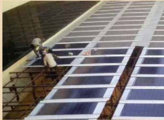
Solar Embedded roof
