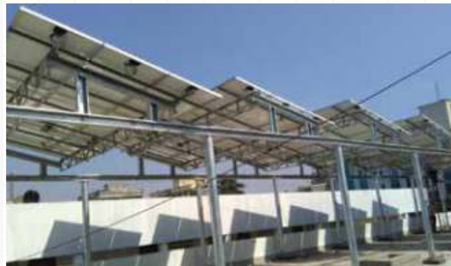
30Kw elevated power plant in Pune
