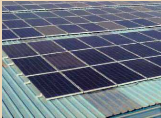
Conventional Solar on Roof
