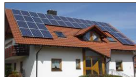
Off-grid home solar system
