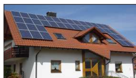
Off-grid home solar system
