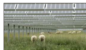
Farm solar generation system
