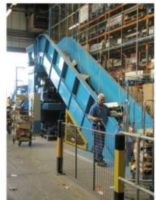
End on view of the Southern Co-op installation.
